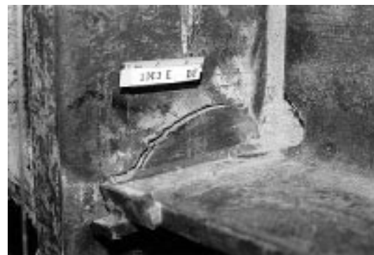
b. Column Flange “Divot” Fracture
