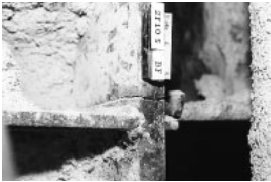
a. Fractures through Column Flange
