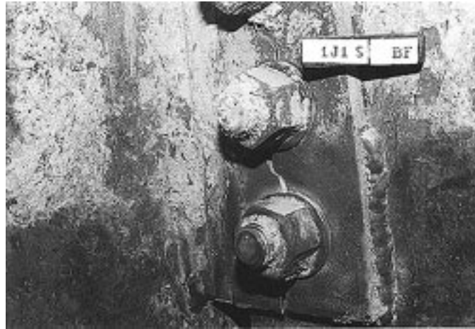
Figure 1-4 - Vertical Fracture through Beam Shear Plate Connection
