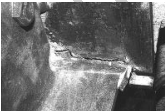
a. Fracture at Fused Zone
