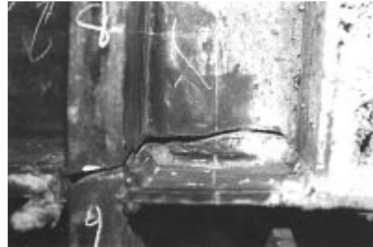
b. Fracture Progresses into Column Web
